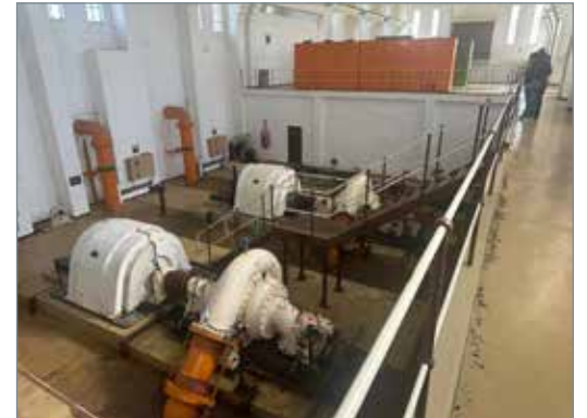
Critical Water Pump Station in the Free State where two FBL 500-400 Double Suction Split Casing Pumps have been in operation since 1967. They were built in South Africa and regularly maintained
