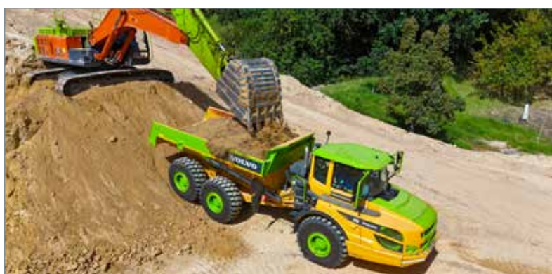
A Volvo A30G articulated hauler being loaded on a site where Hamilton Plant Hire is currently executing a major bulk earthworks and civils project for a new housing development.
