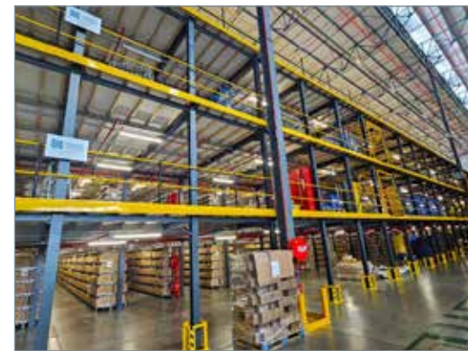
One of the many multi-level GMS systems installed in South Africa.
