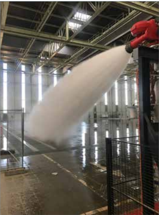
For recycling facilities, the ability to detect abnormal heat and respond before flames develop can reduce the potential for major fire damage and operational disruption.
