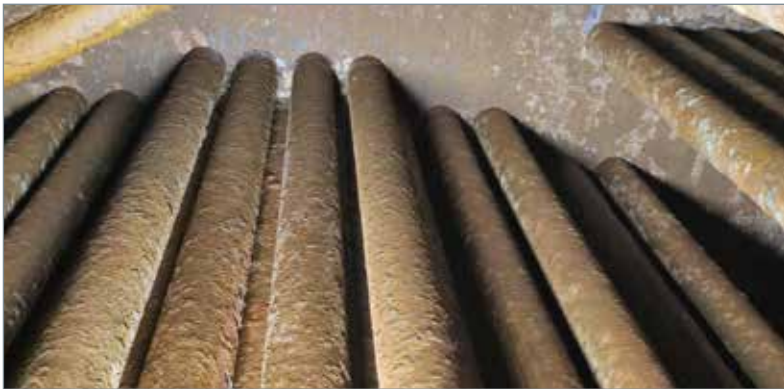
Following Allmech's boiler water treatment at the Warmbaths Forever Resort, there was less corrosion in the boiler and less scale detected on the inner tubes.
