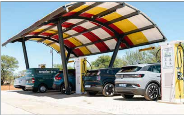
CHARGE's EV charging station in Wolmaransstad
