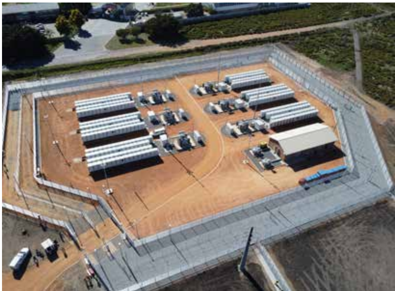
Eskom's Battery Energy Storage System (BESS) project site at Worcester
