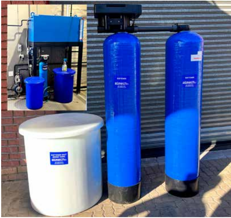
When water treatment and softener systems are planned, supplied and managed as an integrated solution, businesses can reduce operating costs, minimise downtime and benefit from clear accountability throughout the system.
