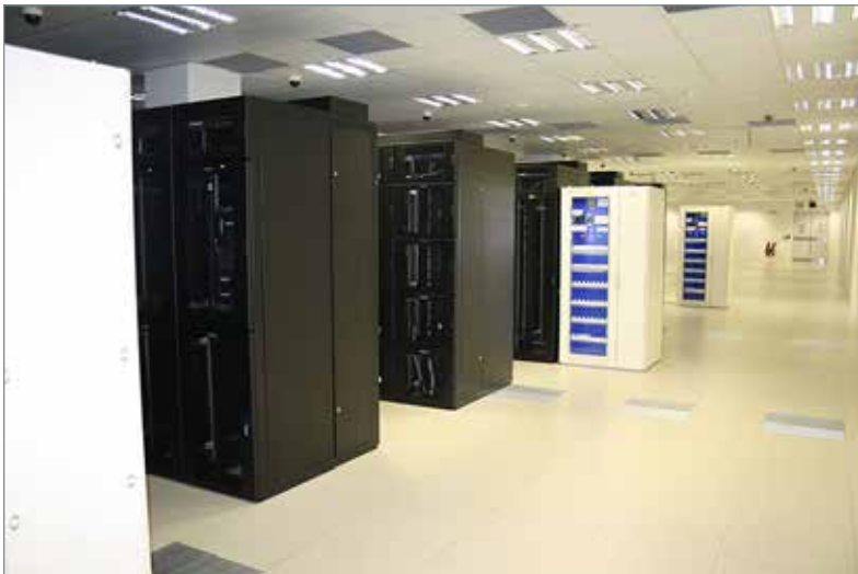
Inside Vodacom Cape Town Data Centre.
