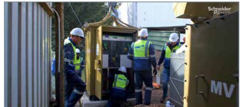
Installation of the Schneider Electric RM AirSeT SF 6 -free medium-voltage switchgear by Technoserve Medium Voltage at Elgin Orchards, Grabouw, Western Cape.
