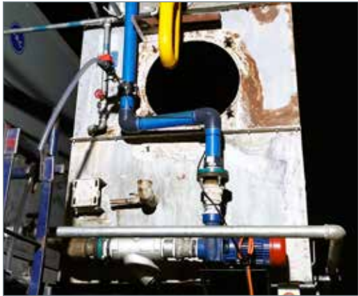
A cooling tower bleed system. Allmech recommends proper bleed control to ensure optimal system performance.
