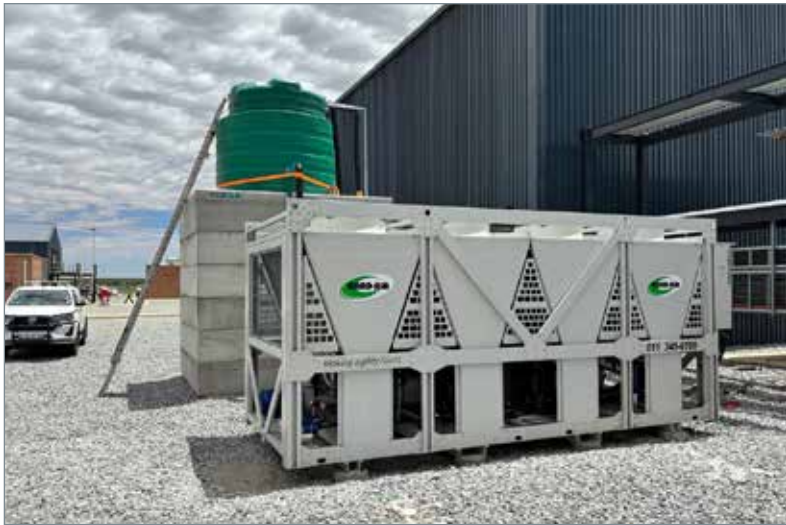
Rand-Air 550kW chiller at a gas plant in the Free State.
