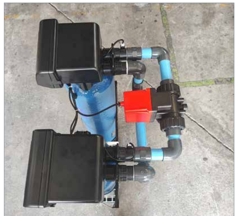
The Allmech duplex water softener.
